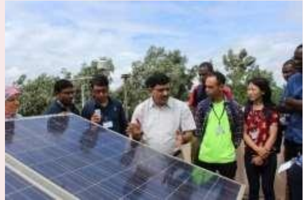
Roof-Top Solar PV System
